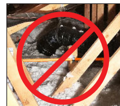
INCORRECT (Exposed piping)
