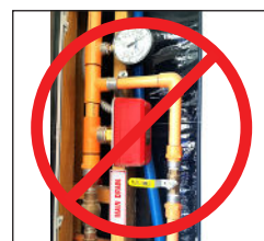
INCORRECT (No pressure relief valve)
